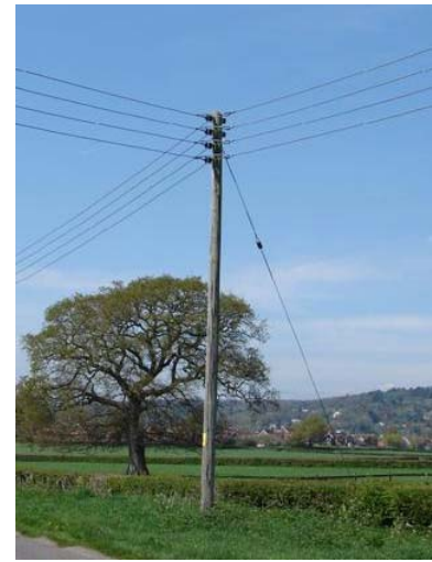
Figure 4 Typical 400 V overhead line open wire (can also be insulated and bundled)
