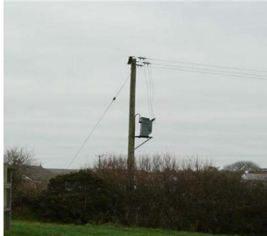
Figure 9 Pole mounted substation
