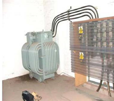
Figure 10 Older design of indoor substation
