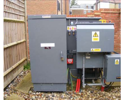
Figure 11 Newer design of compact ground-mounted substation
